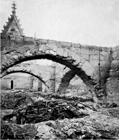
10-20 Reims Cathedral, strainer arches over crossing, exposed after bombardments of World War I.
